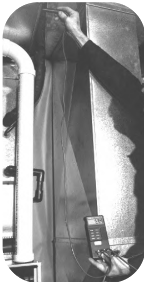
FIGURE 60 TEMPERATURE RISE MEASUREMENT
